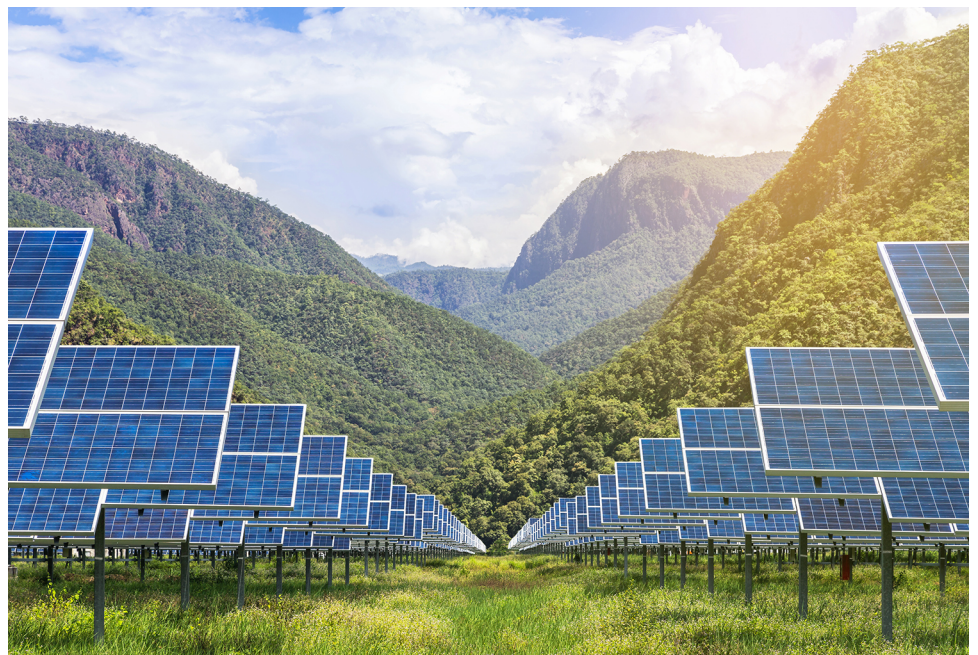
Figure 21. Photovoltaic (PV) panels in sunlight.
